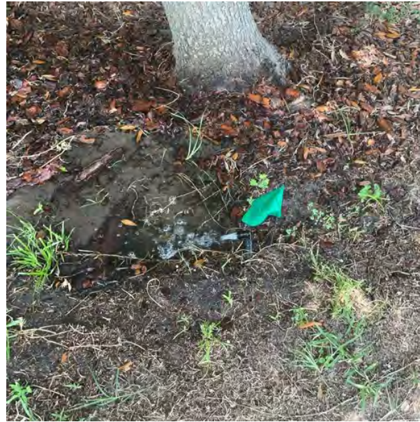
Zone #19 (Broken Lateral) - 08-18-26 1:43 pm CDT
