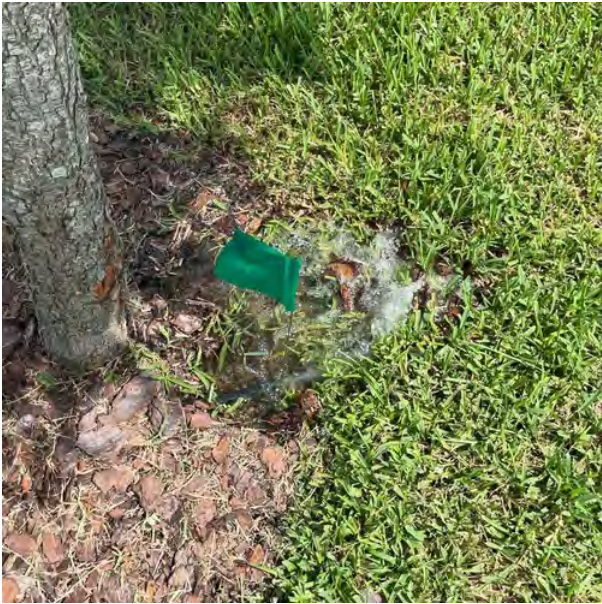
Zone #33 (Broken Lateral) - 08-18-26 2:52 pm CDT
