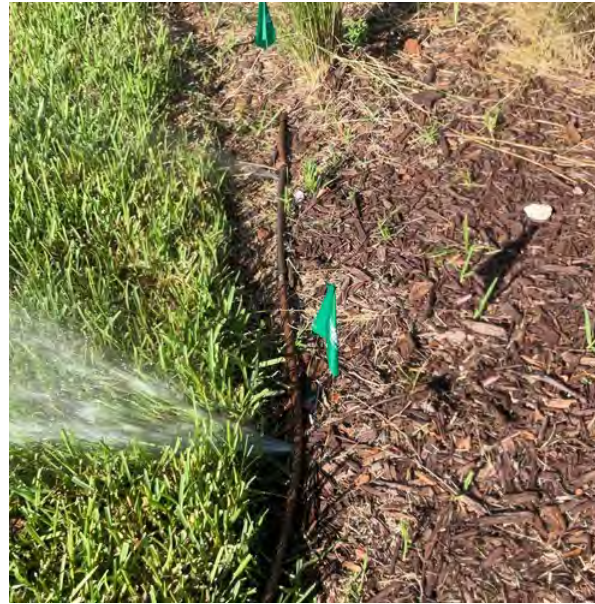
Broken drip 2 different spots
