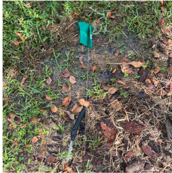
Zone #39 (Broken Lateral) - 08-18-26 3:28 pm CDT
