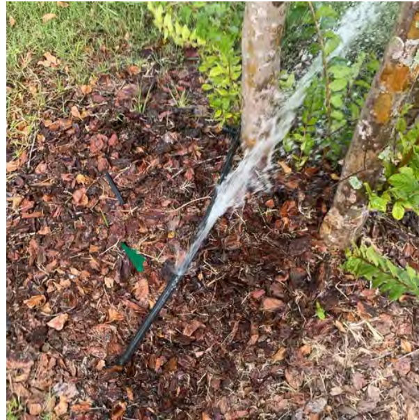
Zone #29 (Broken Lateral) - 08-18-26 2:35 pm CDT
