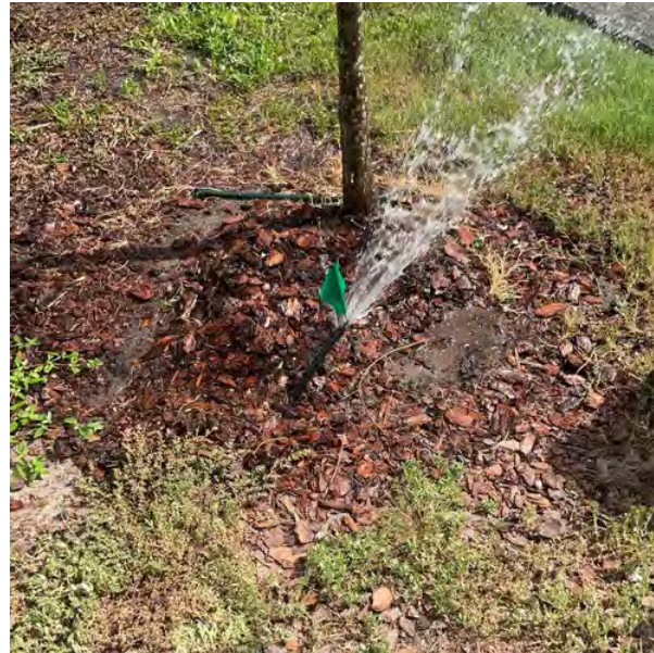
Zone #39 (Broken Lateral) - 08-18-26 3:28 pm CDT
