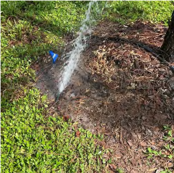
Zone #39 (Broken Lateral) - 08-18-26 3:28 pm CDT
